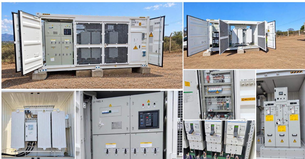
Smart Transformer Station (STS) 3.300 kVA del PSFVC Villa General Belgrano
